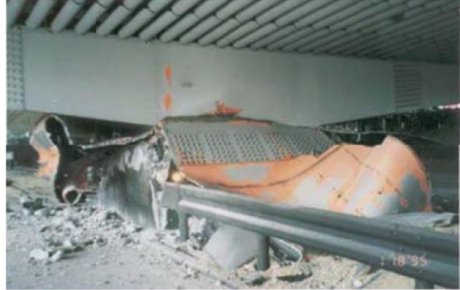
(b) Full Collapse.
